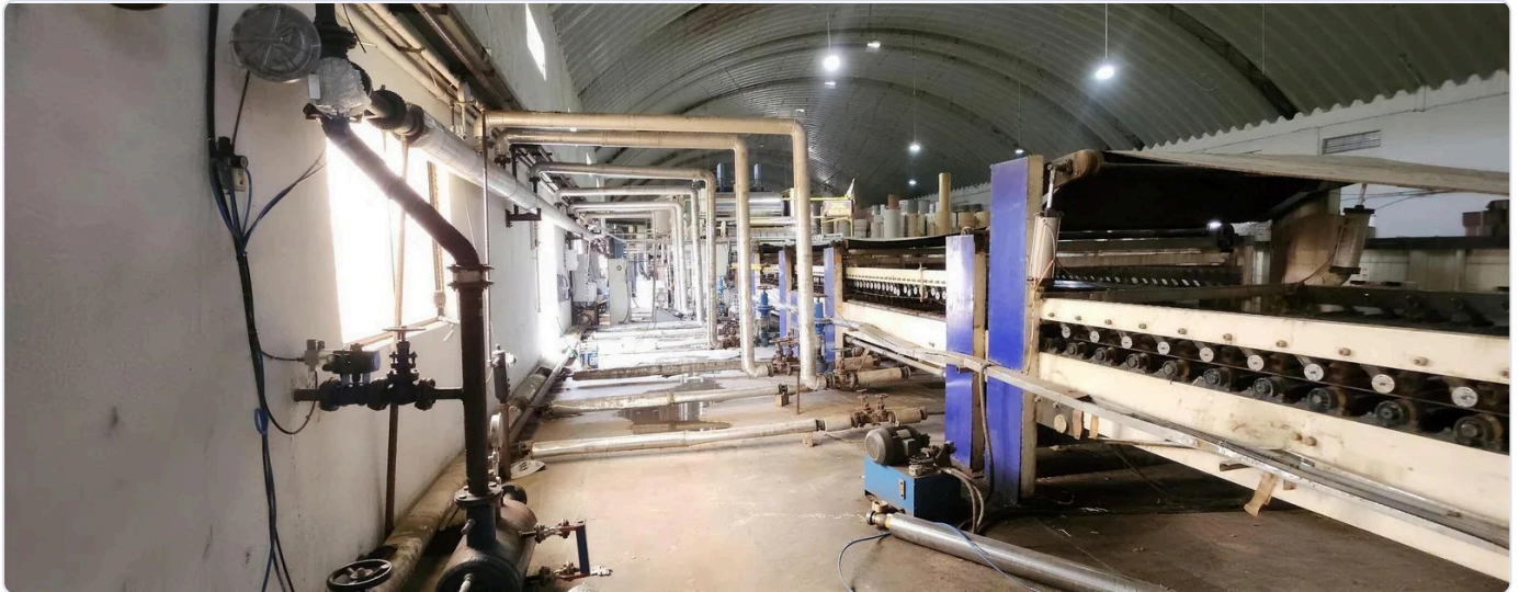
The corrugator line after the Jetomat TurboHeat® steam-system retrofit.
